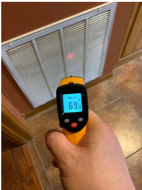
Return air temp
