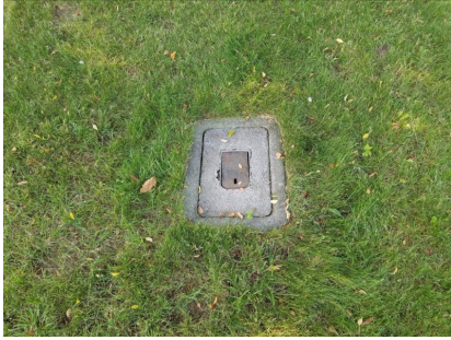
Main Water Shutoff Valve
