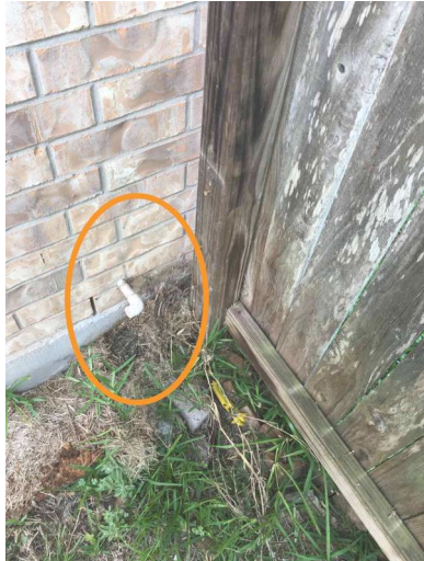
TPR valve drain facing the wrong direction
