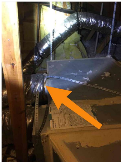
Disconnected support strap
