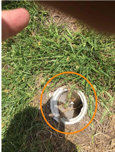
Sewer cleanout missing cap
