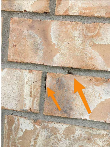
Gaps in mortar
