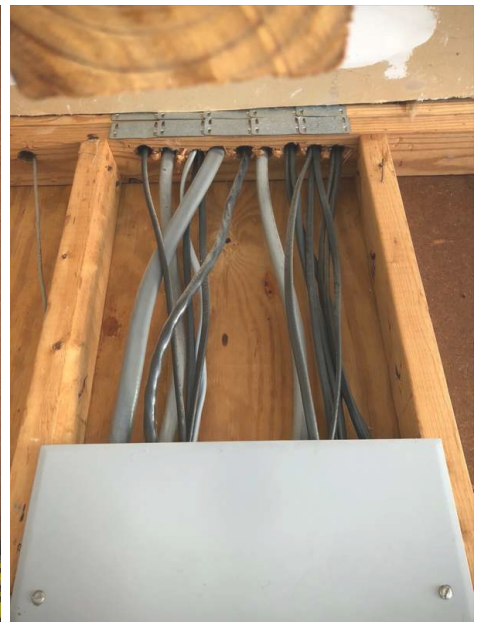
Recommend concealing wires for safety purposes
