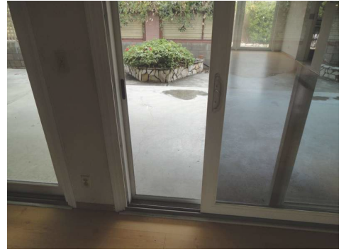
missing screen Dining Room
